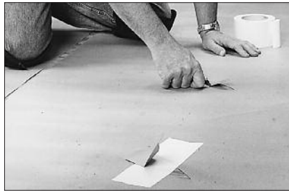
Cut windows in the paper to expose the subfloor and then use masking tape to hold the paper in place. Paper should be rough-trimmed using a utility knife to 1" from all obstructions.
