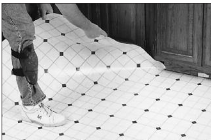
Now that the transfer and cutout are complete, the material is ready to be installed. The floor covering is an exact duplicate of the floor, with all excess material removed and all cuts made for possible obstacles. Place the material into the room and fasten as required.
