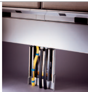
Base power in-feed conceals conduit from floor to main beam.
