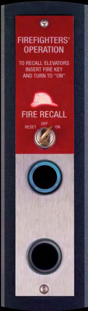
Intermediate Hall Station with Fire Service Devices
