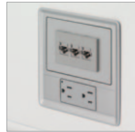
Technology skins provide convenient access to power and data.
