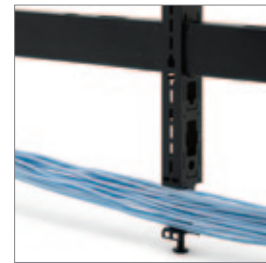
Ample space in the base area supports lay-in of cabling.
