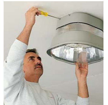
...and secured to the j-box assembly with a very secure lift, shift and click motion.
