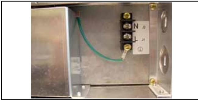
Figure 7. Junction Box Wiring
