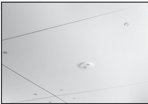
Front View of Installation for Heat Sensor
