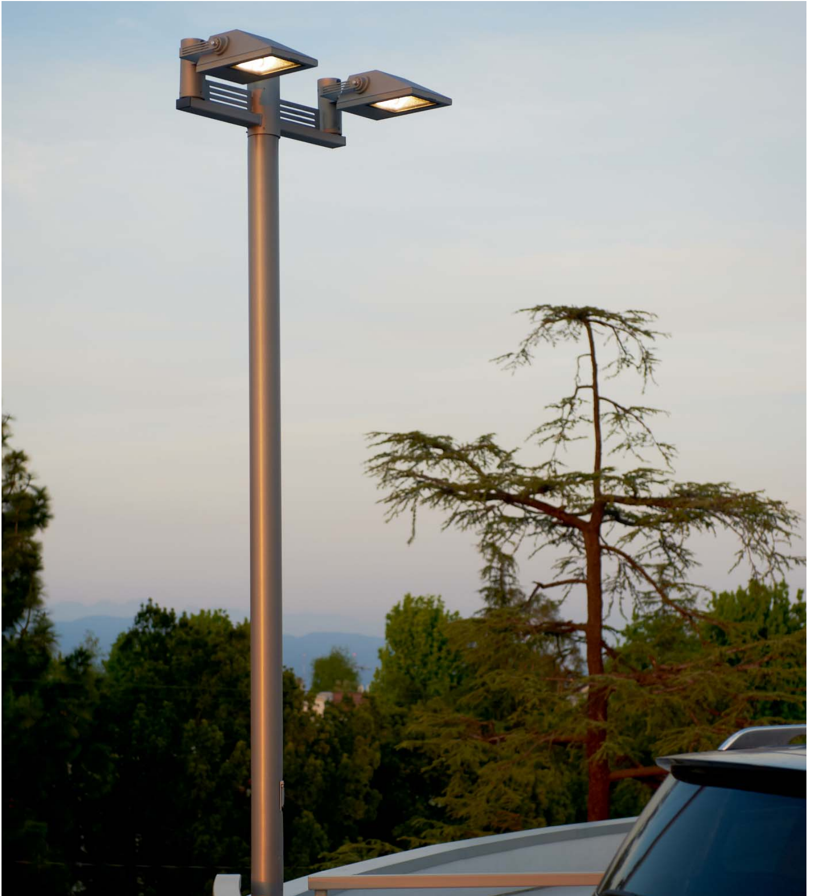
Keyes European Van Nuys Expansion. Van Nuys (USA). Architect: Dennis Flynn Architects, Inc. Lighting design: Lighting Design Alliance.
