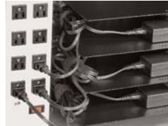
Built-in power supply
